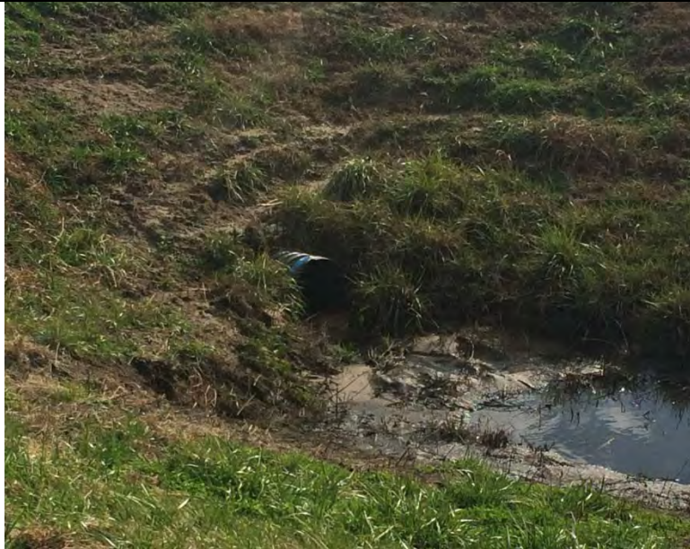
Photograph No. 9 AECI UWL Inspection Stormwater pipe from drainage ditch to sedimentation pond
