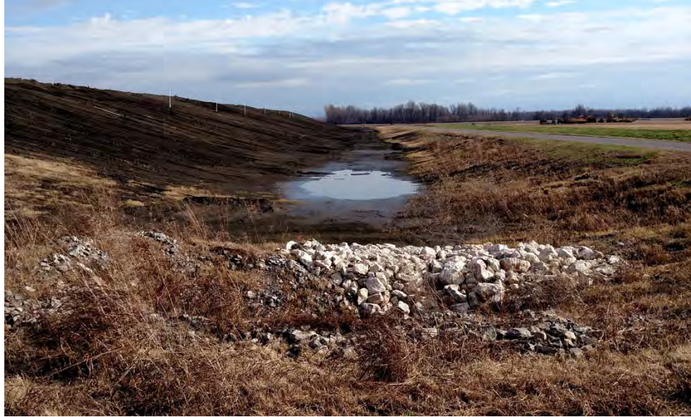
Photograph No. 5 AECI UWL Inspection Southern landfill face and rock protection at stormwater pipe
