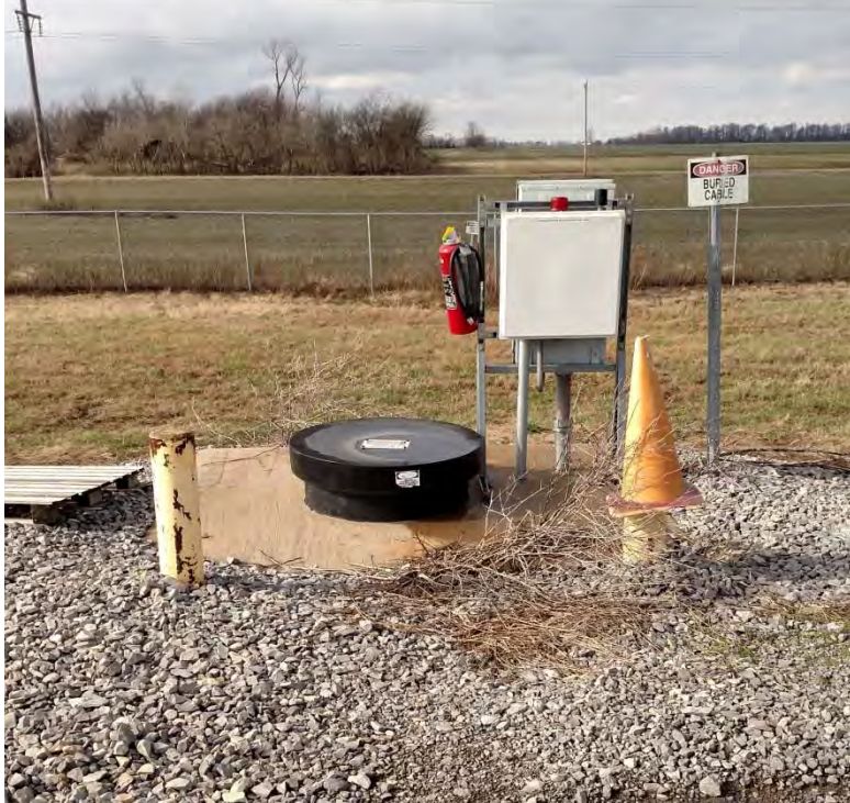
Photograph No. 3 AECI UWL Inspection Inspection leachate collection manhole cover and electrical control box for pump
