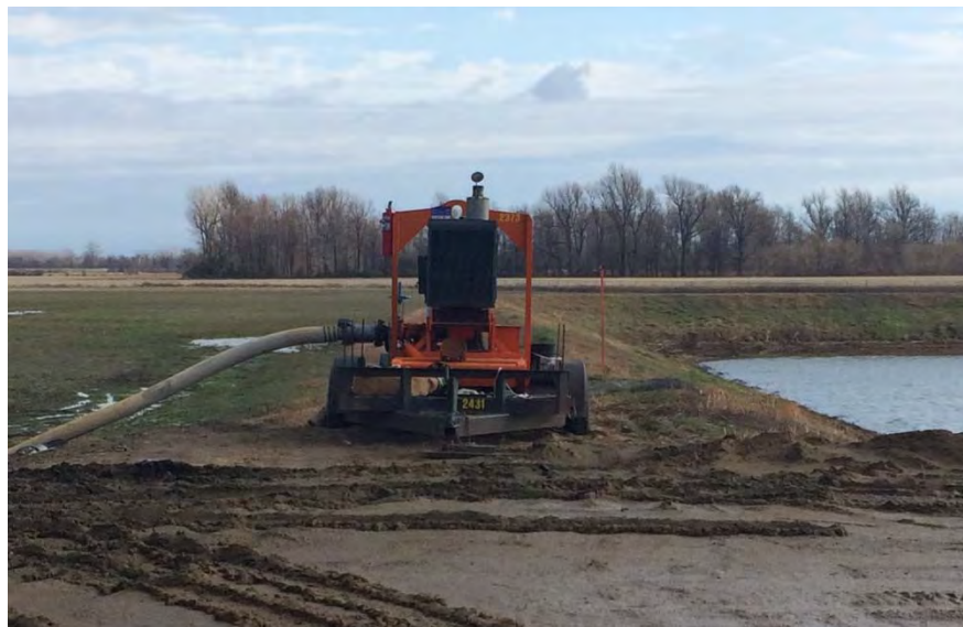
Photograph No. 10 AECI UWL Inspection Mobile pump unit, pumping from sedimentation pond
