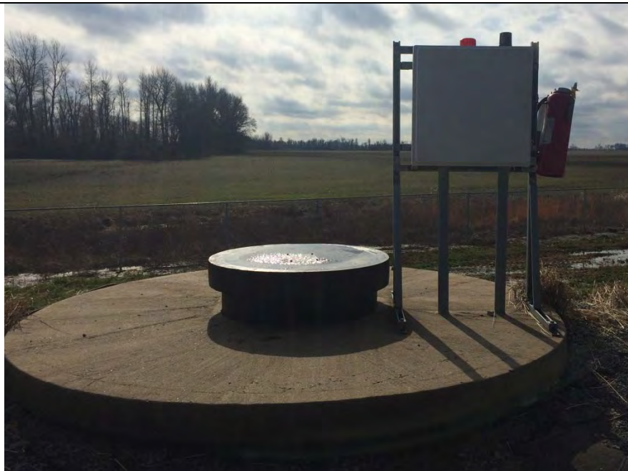
Photograph No. 16 AECI UWL Inspection Leachate loadout pump structure cover, electrical control box for pump
