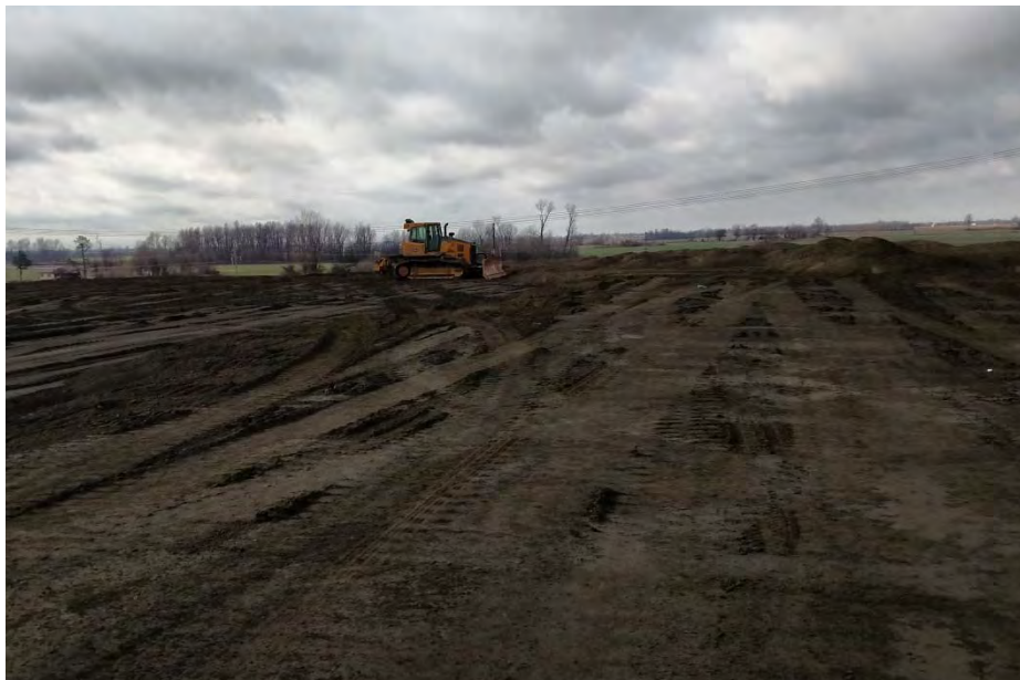
Photograph No. 12 AECI UWL Inspection Top of landfill; bulldozer used for CCR grading
