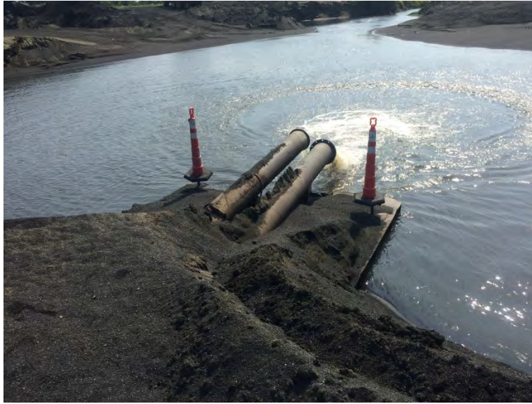
Photograph No. 1 Pond 003 - two inlet pipes
