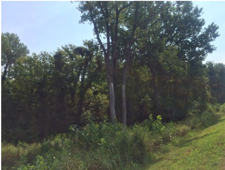
Photograph No. 4 Pond 003 Dead trees at downstream toe of eastern embankment
